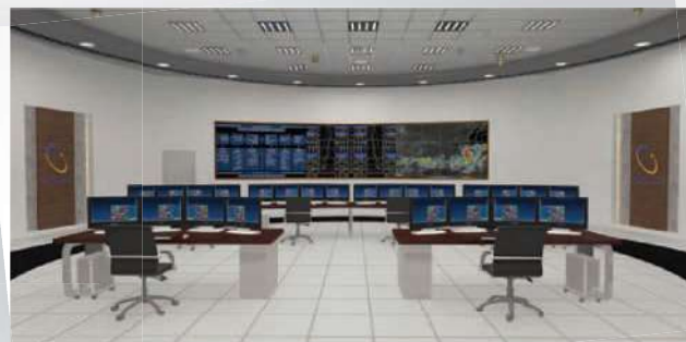
Scada Control Room View1 Jeddah LDC Upgrade and DMS
